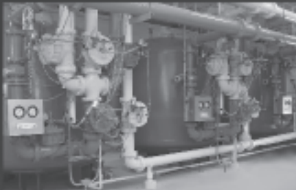
Radium and Iron Removal Systems
